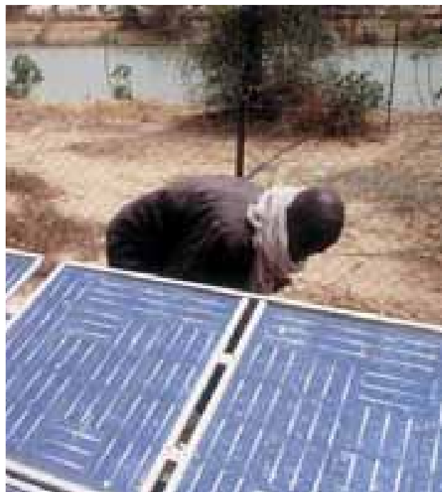
Solar panel for the operation of a water pump, Senegal
